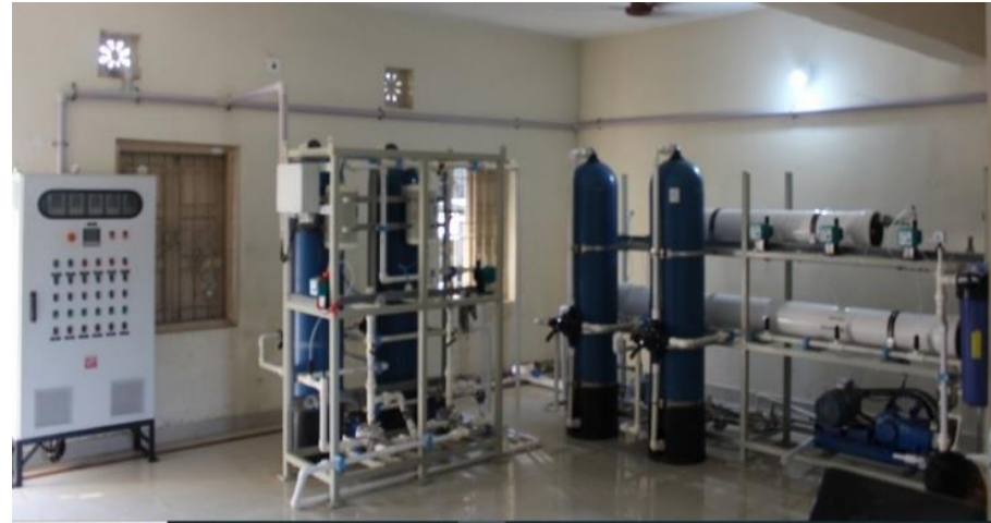
Batch RO- FO unit at School (capacity 800 lt/ hr, recovery 80%)
