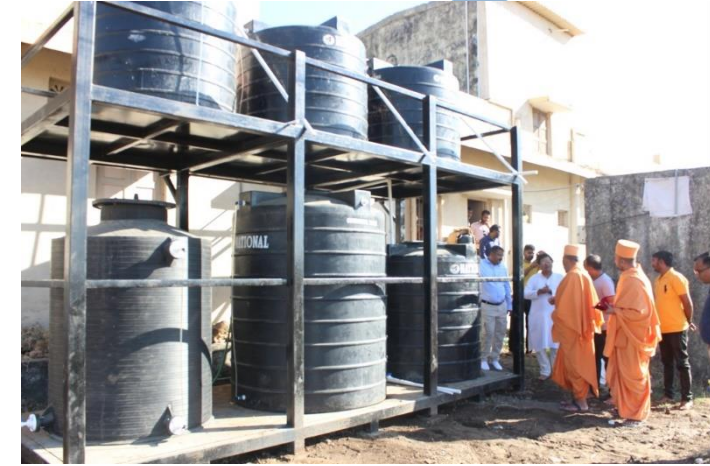
Water tanks outside the machine room
